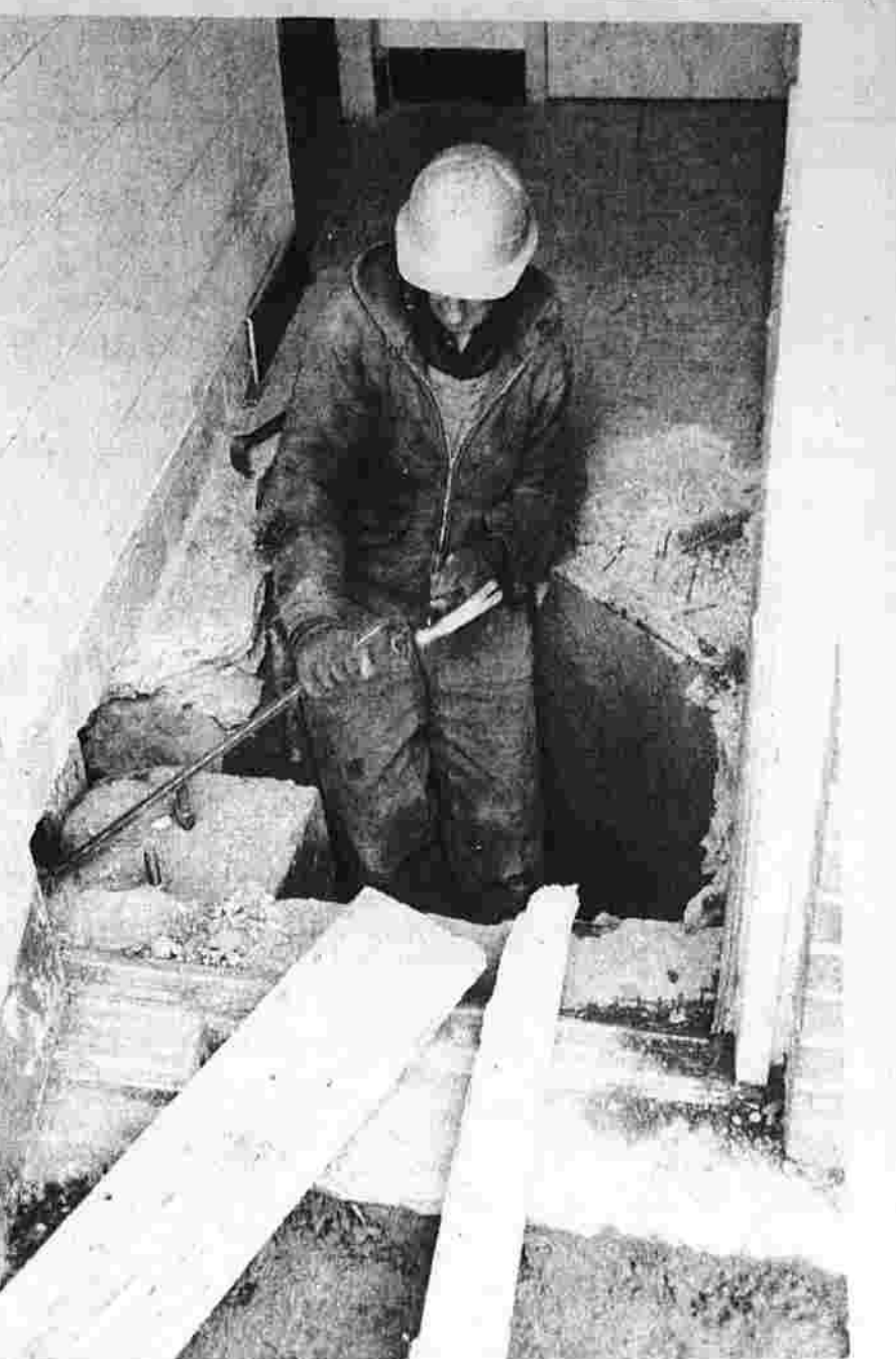
Joining the Old with the New, Larry Cyr stands in a hole in the boys' locker room at Illing Junior High School while stripping planks away from the foundation in order to connect the old foundation with the new one of the construction project presently under way. The new addition houses a two-story gymnasium and additional classrooms. (Herald photo by Dumm)
